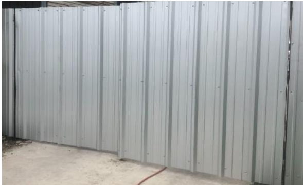
Unpermitted Unframed, Untreated Corrugated Metal Fence
