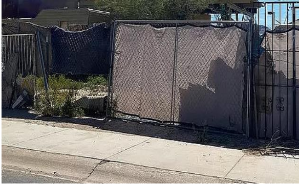
Unpermitted Multi-Material Fence
